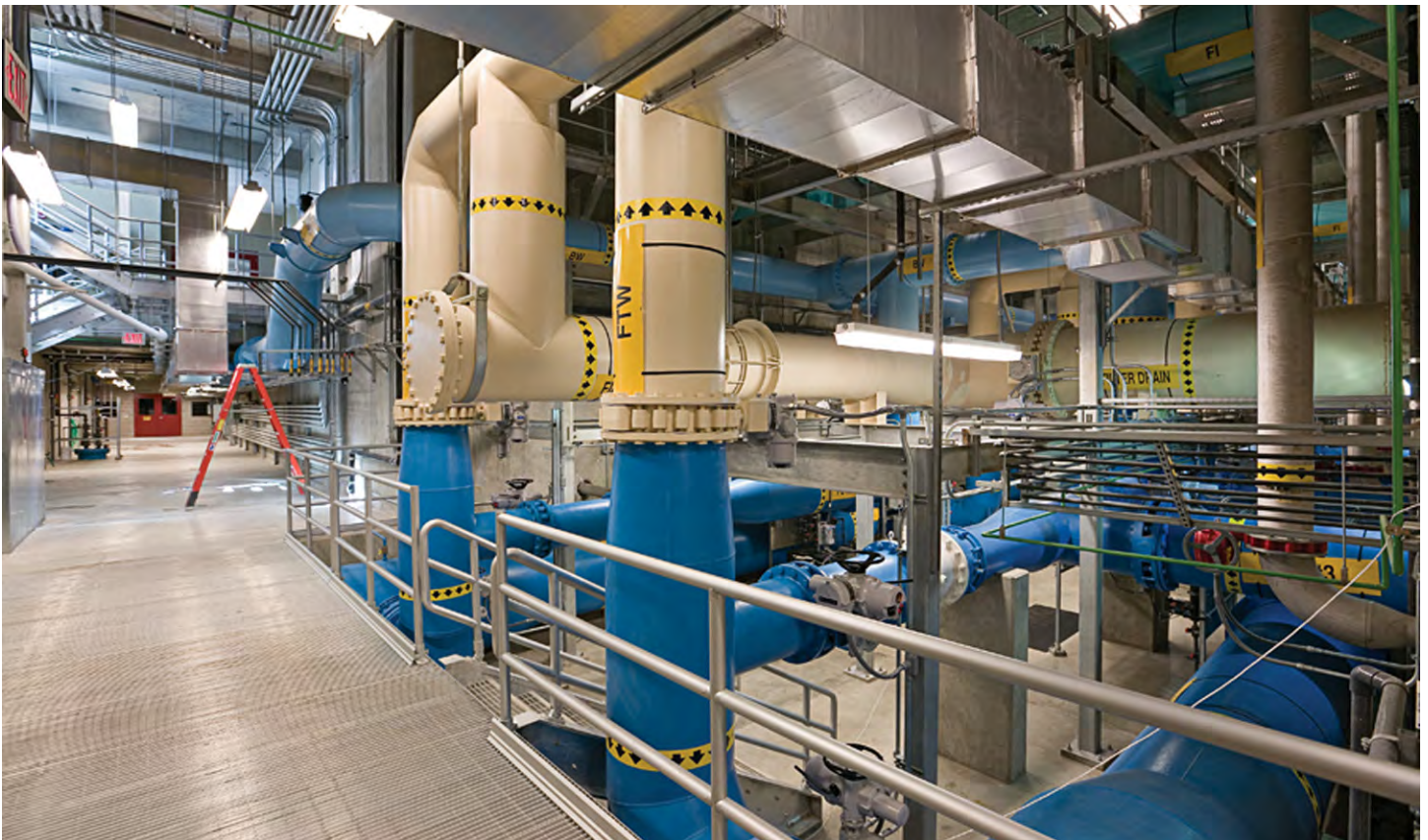
Nelson-Flanders Water Treatment Plant Longmont, Colorado
