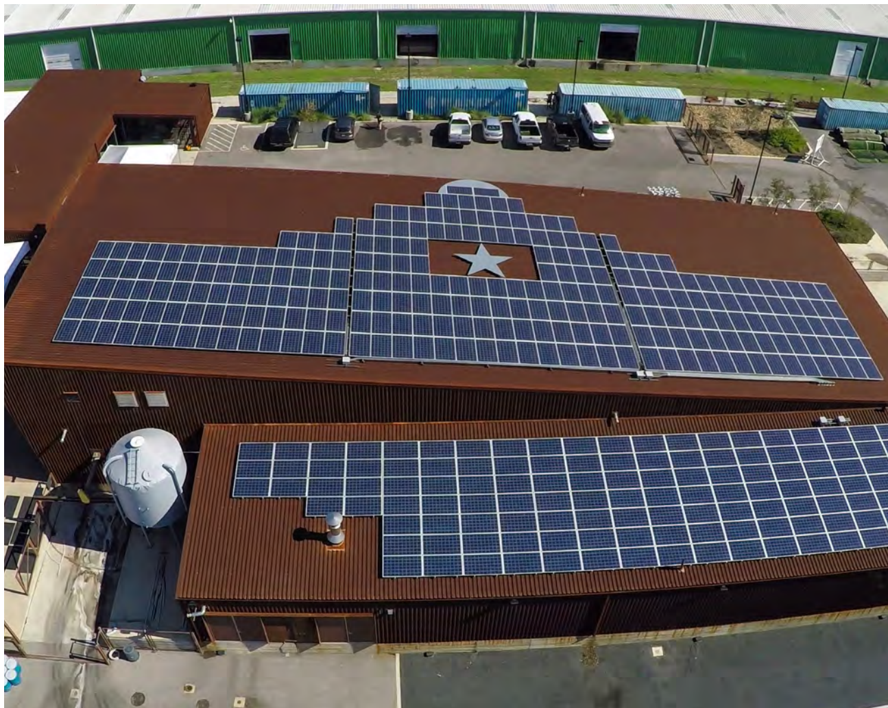
Photo courtesy of One80 Solar
